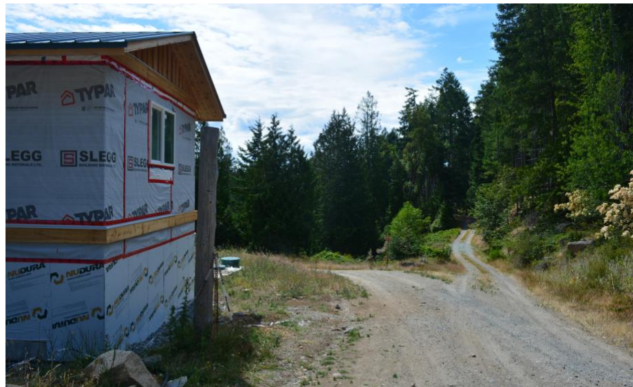
View looking down the hill. The Program Centre is on the left and the channel to be used as the course of the bioswale is visible between the side of the building and the road. The bioswale will follow the curvature of the road, hugging its left side. Photo: Adam Dewar
