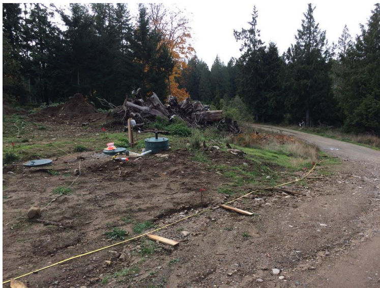
Figure 7.3.1: Marked perimeter and terraces of the bioswale on Site A before machine work day
