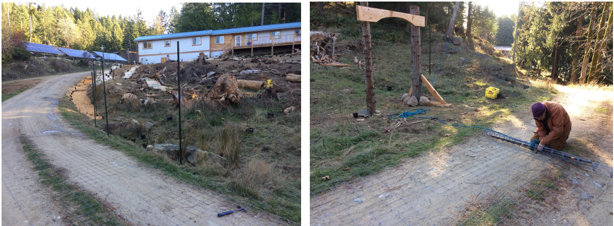
Figure 7.3.1: Fencing is laid out along the road to be erected onto metal poles at Site A
