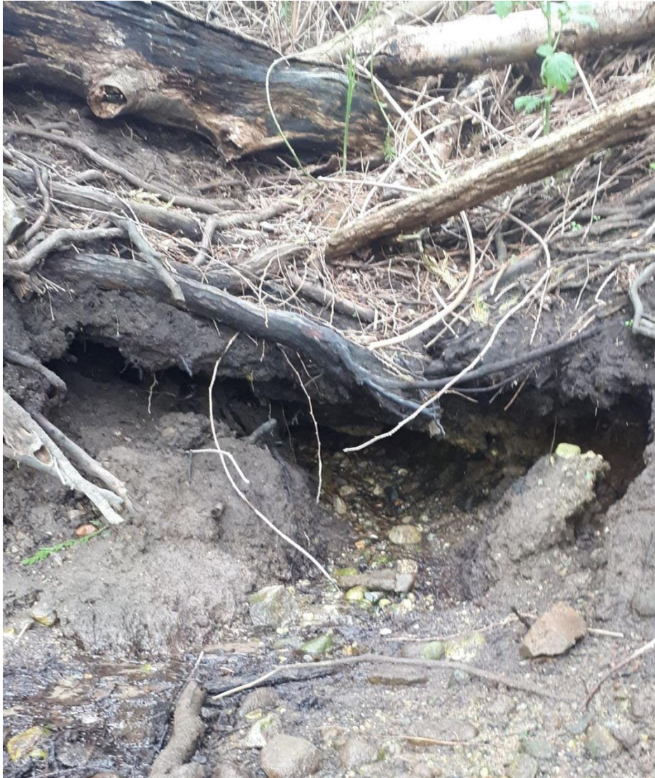
Figure 24 The creek that feeds in Whaler Bay, reappearing from where it was diverted under the road.
