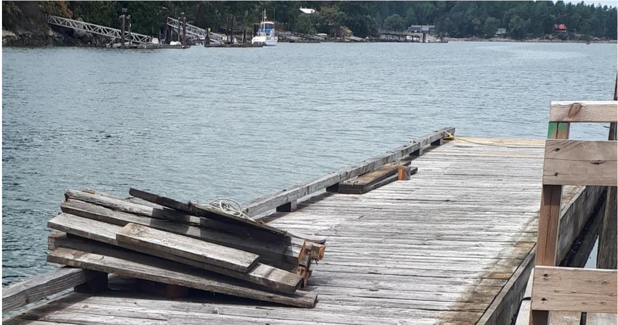
Figure 17 A public dock piled with treated wood is evident in the foreground of this picture of Whaler Bay, while various residential docks and vessels rest in the background.
