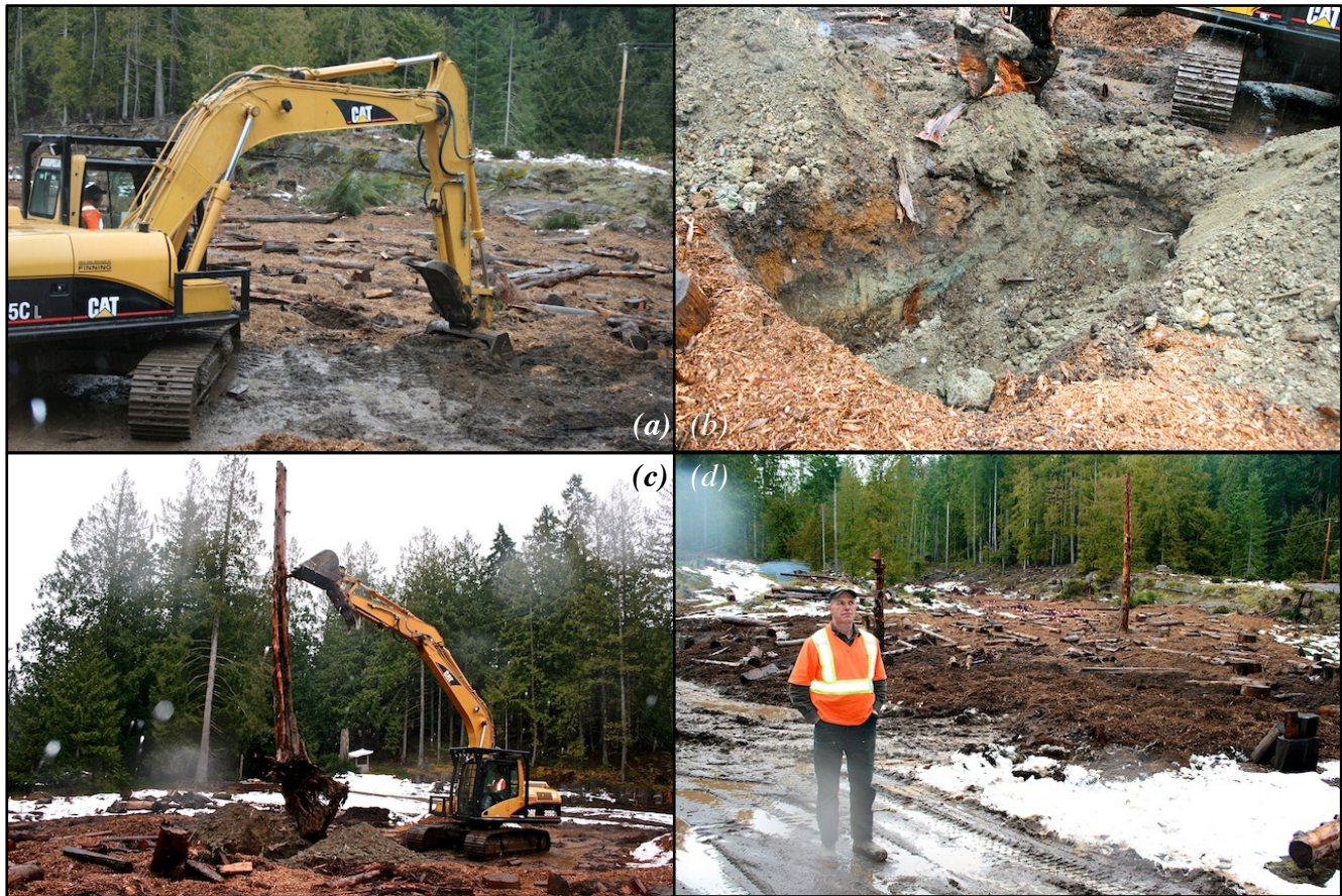
Figure 8. (a) Rough and loose de-compaction, with the excavator bucket reaching about 1m in depth; (b) 2m-deep pit dug for anchoring a snag in the ground. Considering that pools of water were covering the soil surface, the absence of water in the excavation confirms that there was very little subsurface percolation, probably due to a combination of anthropogenic surface compaction and the natural occurrence of a restricting layer, the blue clay horizon visible at mid depth; (c) a 15m-tall snag being installed in the ground; (d) proud excavator operator Fred Stevens, ‘hero’ of the day (photos taken on March 4 th , 2014)
