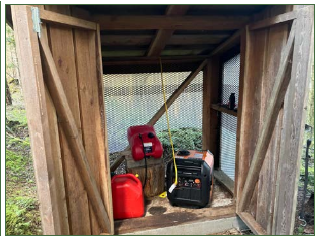
Photo 10 - Generator shed (GAIA)
