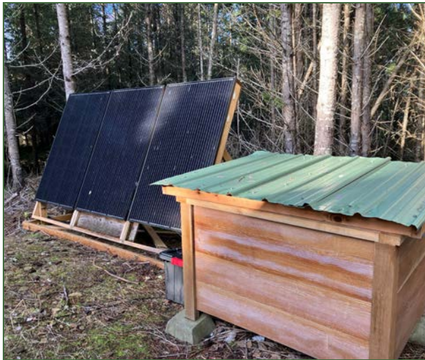
Photo 11 - Solar Panel and battery shed (GAIA)
