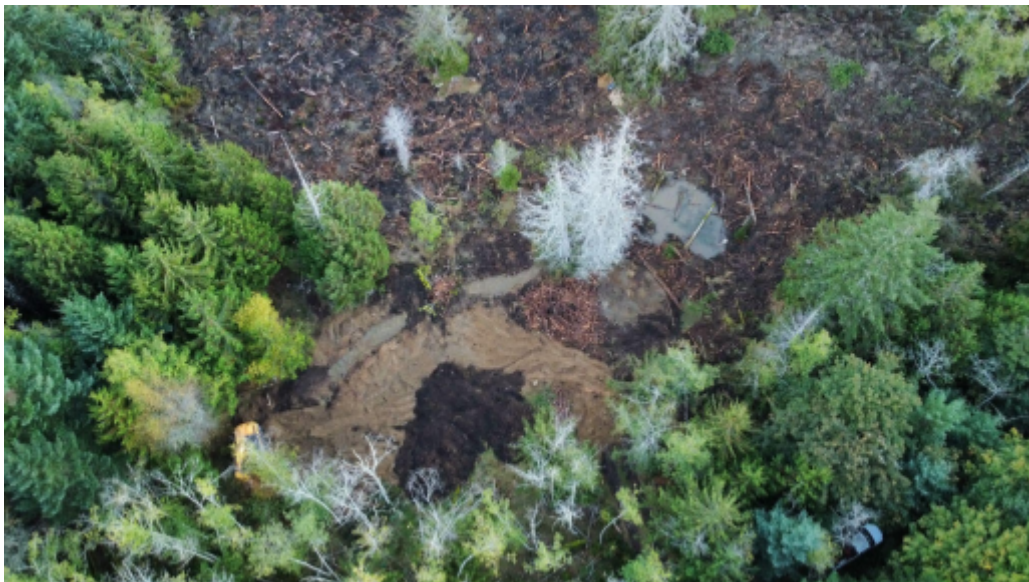
Figure A2: Construction underway on the final wetland and core trench features for the project
