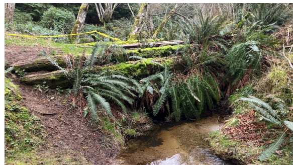
Figure 4: Failing earthen road crossing, Mar. 2025
