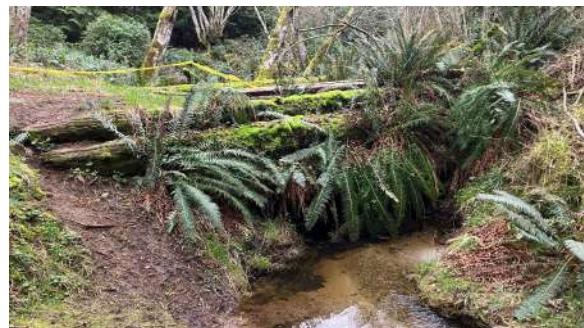
Figure 4: Failing earthen road crossing, Mar. 2025
