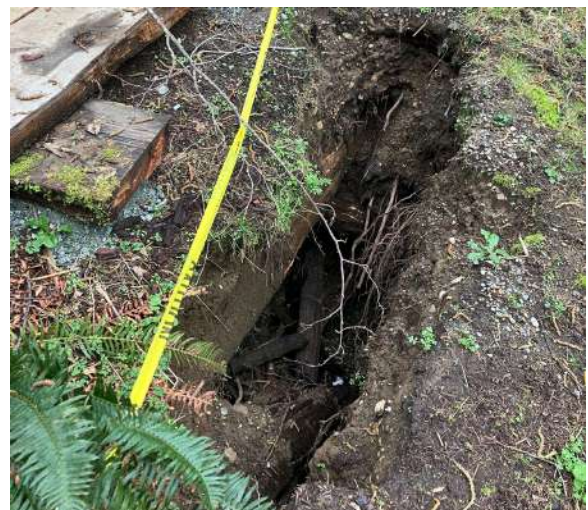
Figure 10: Sinkhole forming in Crossing #1, 2025
